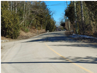
South End, Facing north, S bend, one of many blind spots, 40kms
