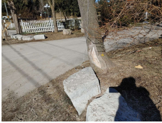
North End, Facing north, S Bend. Damage left from car collision, right where children wait for school bus, 40kms
